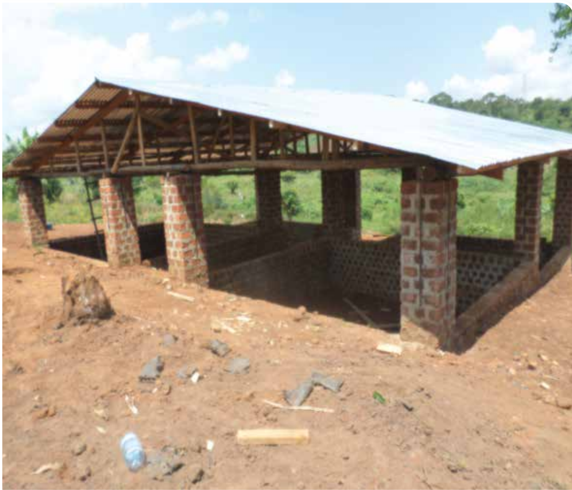
Figure 20 four unit FBT piggery housing structure before plastering of walls was done.
