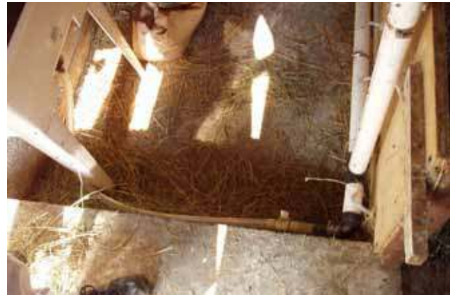
Photo 3.2 A flexible tube with a valve connects the reservoir to a PVC pipe which runs along and is mounted on plywood.
